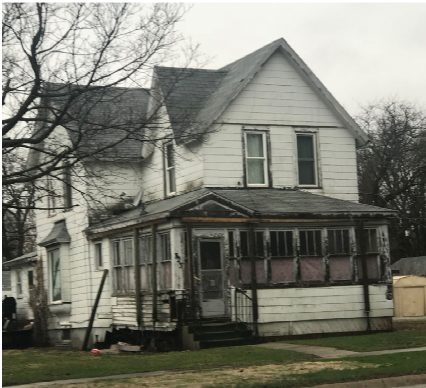
Figure 3 Example No. 3 - Peeling paint, deteriorated windows, and foundation problems.
