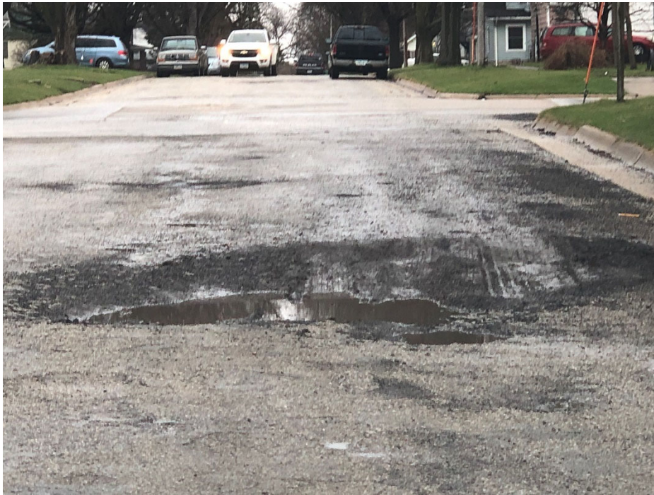
Figure 11 Example of public street deteriorated.
