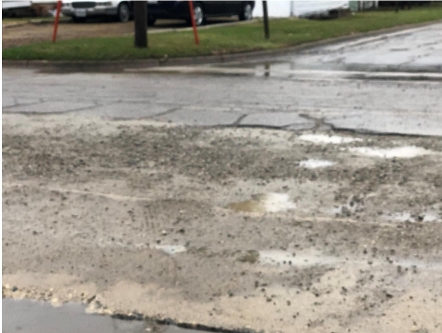
Figure 10 Example of public street deteriorated.
