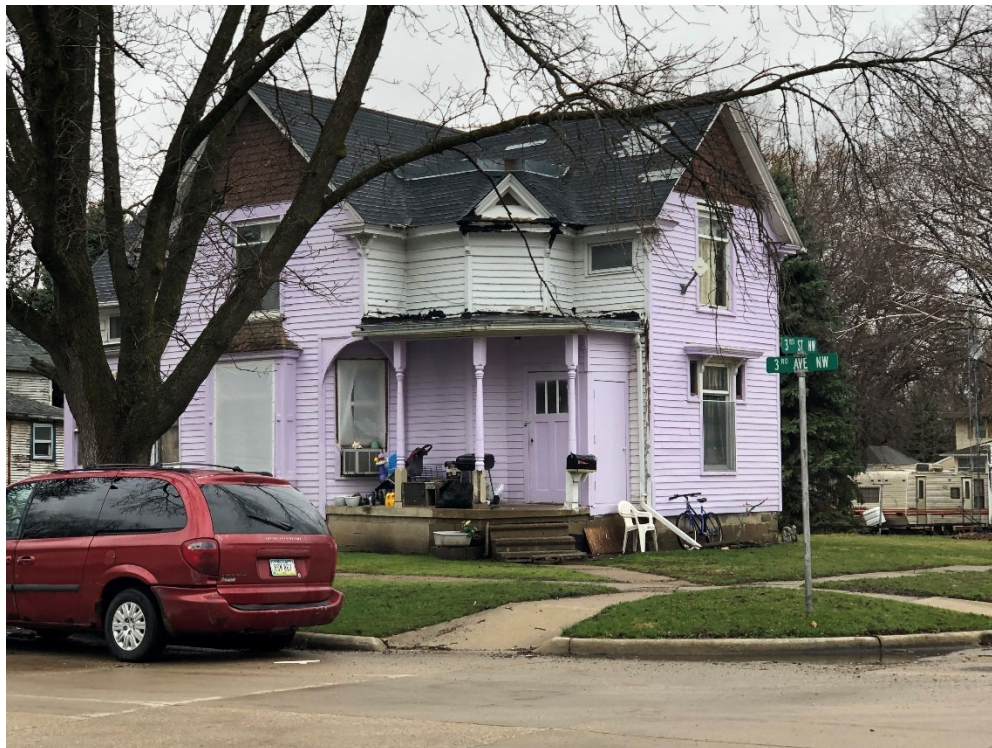
Figure 1 Example No. 1 -Missing shingles, visual blight on and around front porch, and rotten wood.
